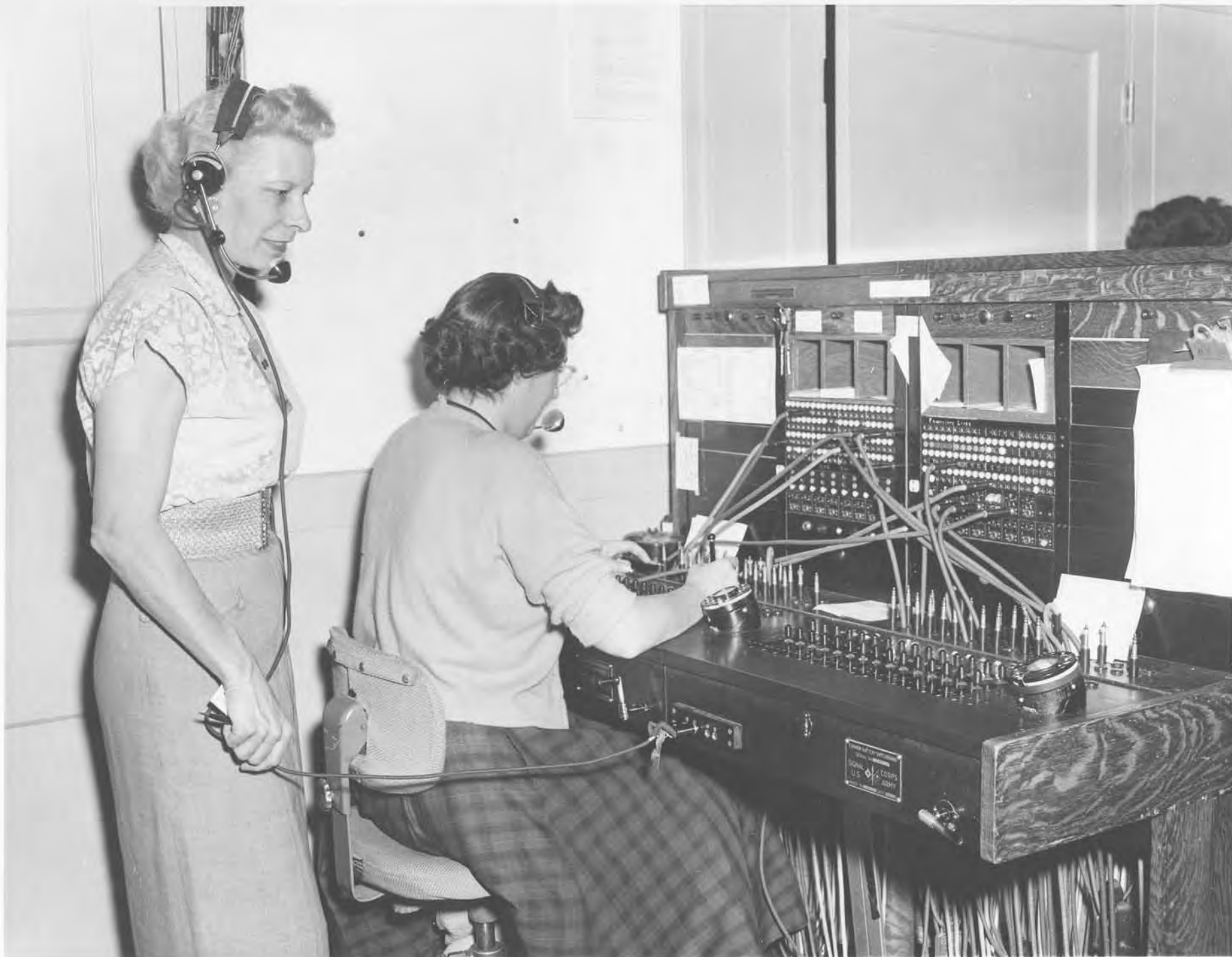
STROMBERG-CARLSON SIGNAL CORPS COMMON BATTERY SWITCHBOARD EDWARDS AIR FORCE BASE, DOUGLAS AIRCRAFT 1955
