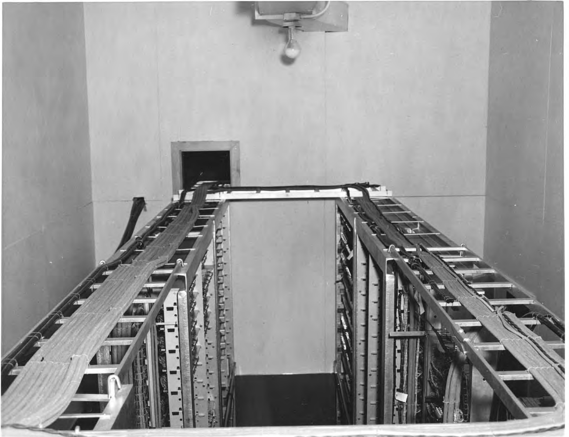
CABLE RACKS WITH CABLES, KELLOGG 7-2 X-BAR, EDWARDS AIR FORCE BASE, DOUGLAS AIRCRAFT, CA 1955
